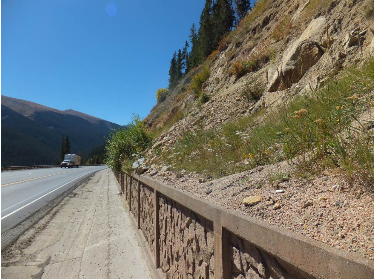
Figure 7-21. Accumulation of sediment on the knee wall and the lower portion of the slope at milepost 237.9
