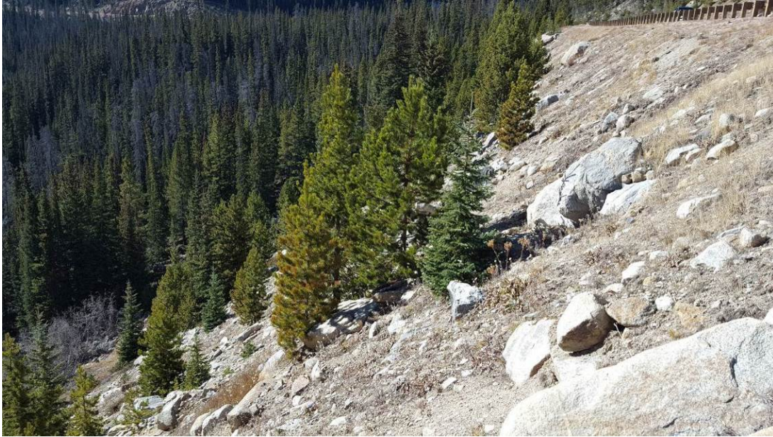
Figure 7-13. Fill side of roadway at milepost 239.1 affected by slope wash and surficial erosion
