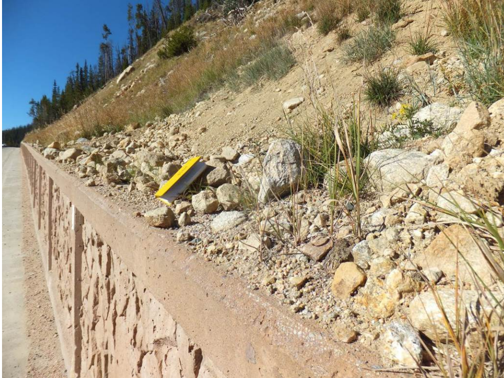
Figure 7-15. Accumulation of slopewash material at milepost 238.7
