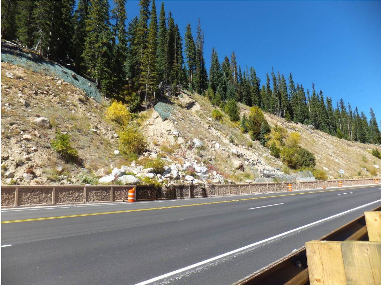
Figure 7-22. Milepost 237.6 showing (A) the glacial till slope (left), (B) active drainage channel with collection of boulders on knee wall (center), and (C) former drainage filled with till and alluvium (right, above damaged Type 4 barrier and fencing)
