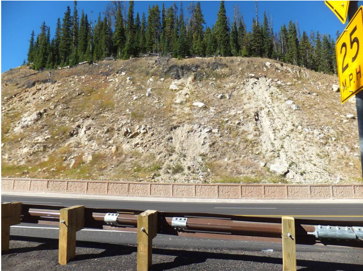
Figure 7-19. Spring blowouts (shallow localized slope failures) and slopewash at milepost 238.2
