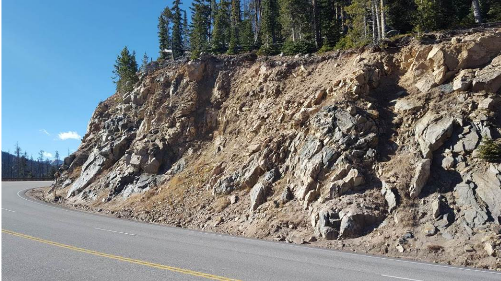
Figure 7-11. Milepost 239.7. Possible shear zone in center of photo
