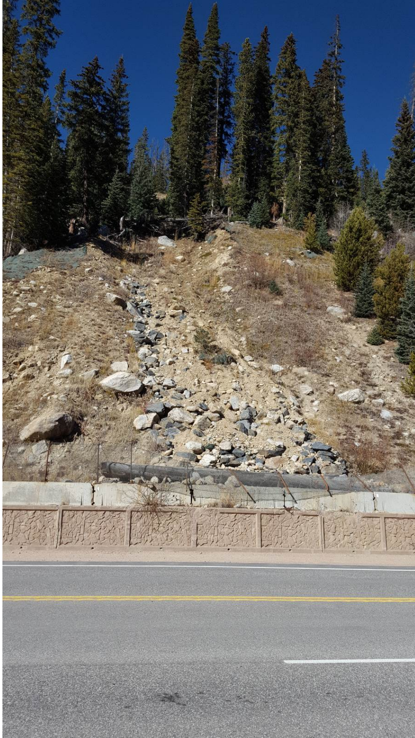
Figure 7-25. Milepost 237.6 C, drainage channel which was partially stabilized with boulders and fill during the mid-90's slope stabilization projects. Type 4 barrier and fencing placed on top of knee wall for erosion and rockfall control has been heavily damaged
