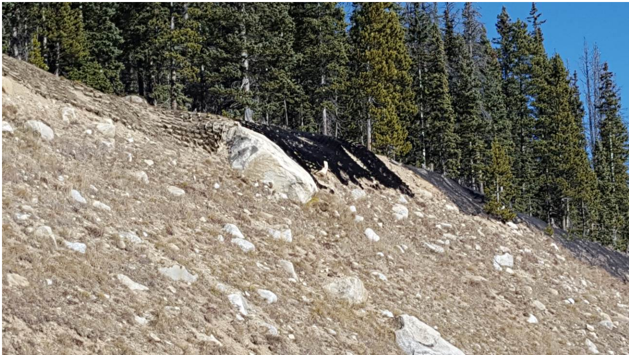
Figure 7-36. Poorly-performing Geocell mats (left and center) and better-performing Enkamat (right)
