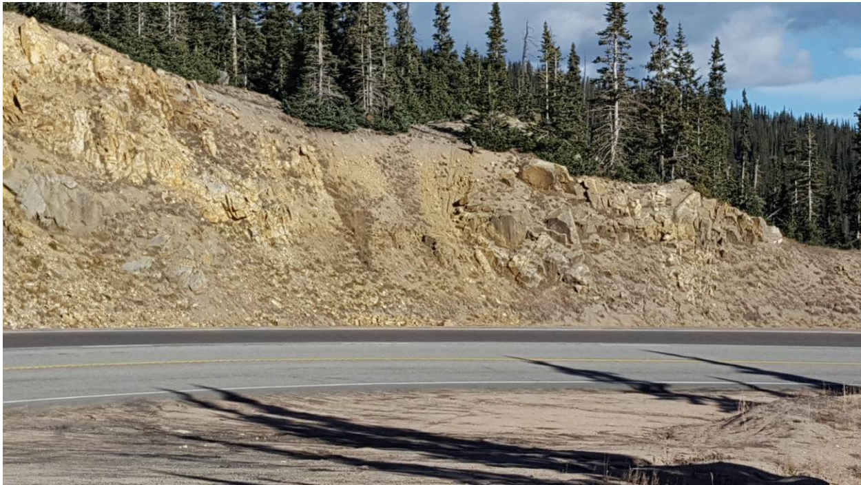
Figure 7-2. Weathered bedrock and possible fault shedding sediment at milepost 242.35 B
