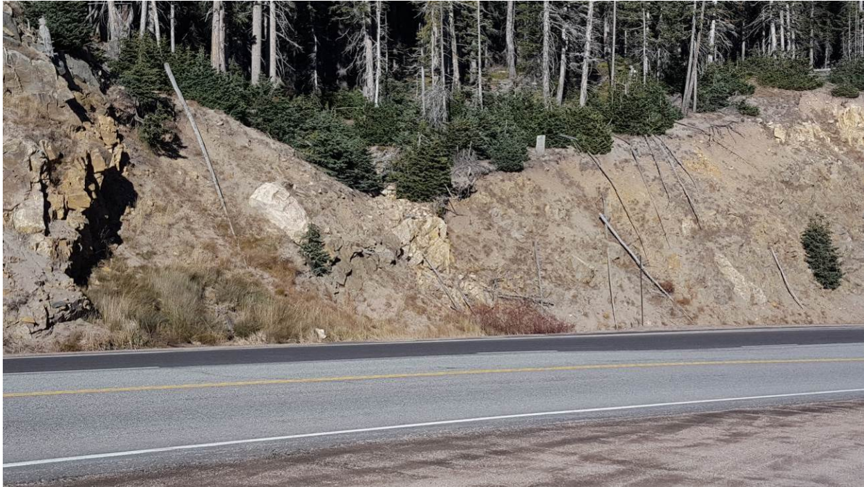
Figure 7-1. Drainage channel at 242.35 A
