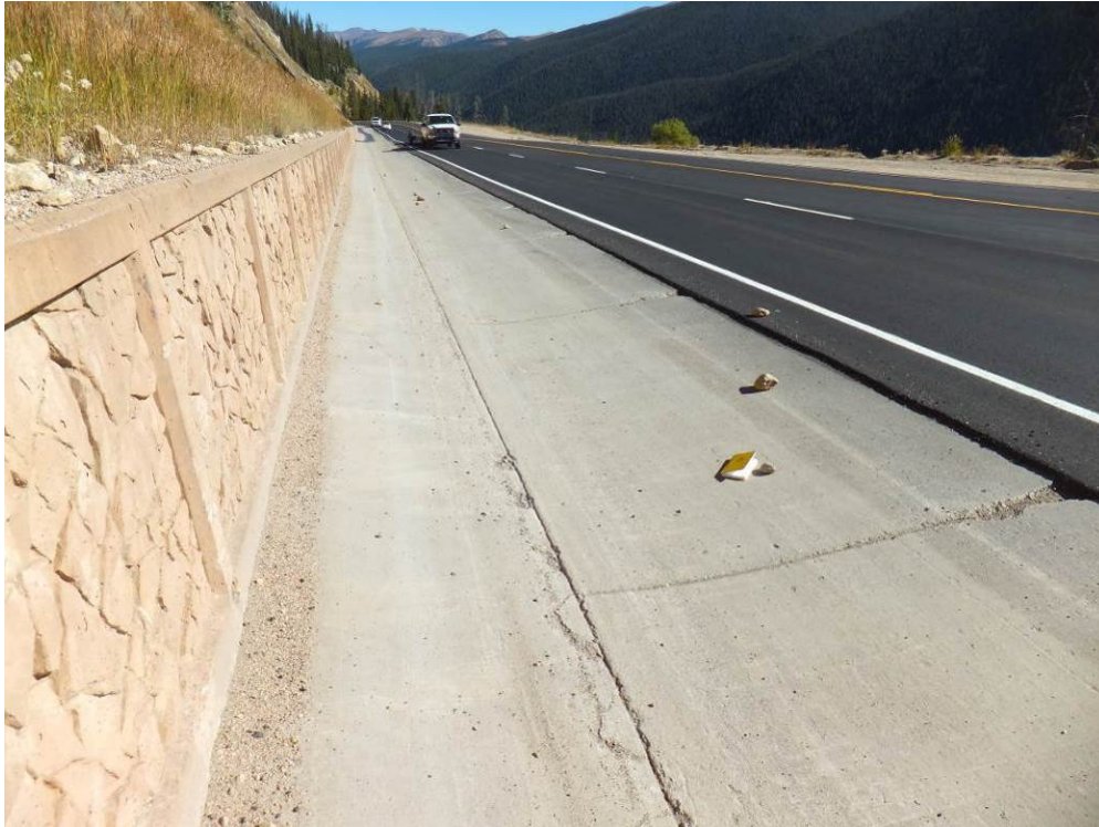
Figure 7-16. Small boulders that have fallen onto the concrete ditch and asphalt roadway at milepost 238.7
