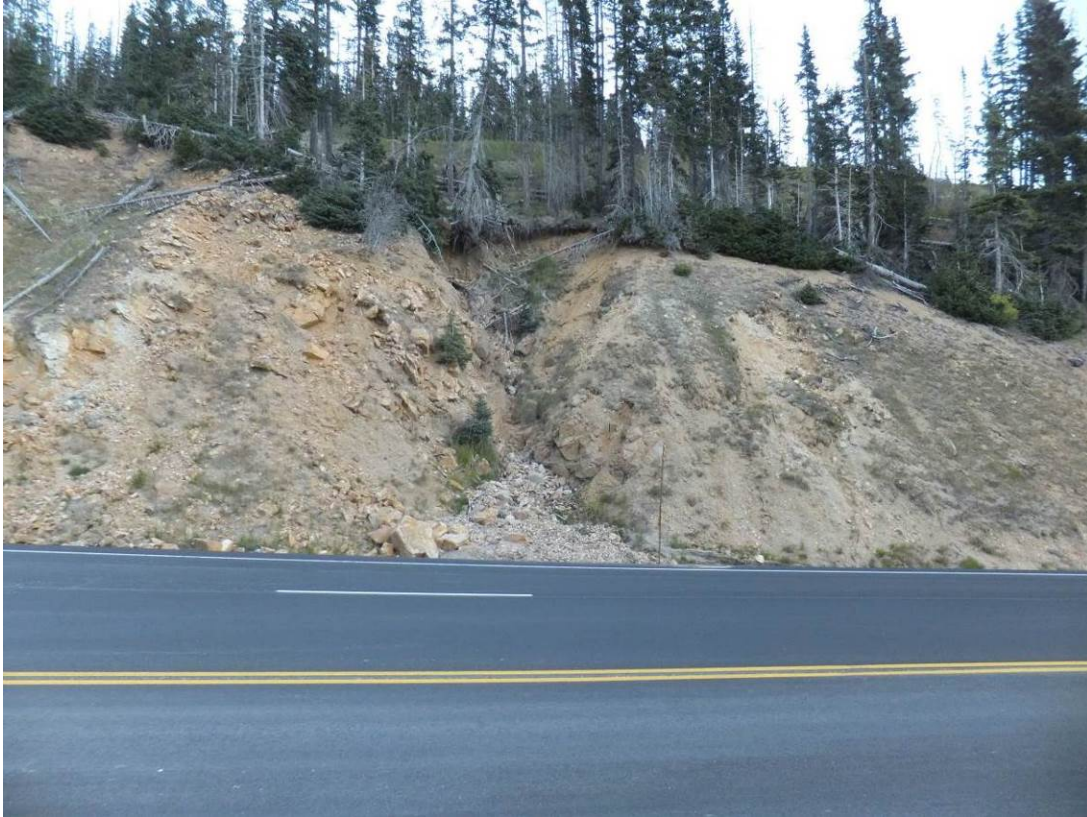
Figure 7-5. Slope failure at exiting drainage at milepost 241.75. Culvert inlet is buried by rocks and sediment at base of failure
