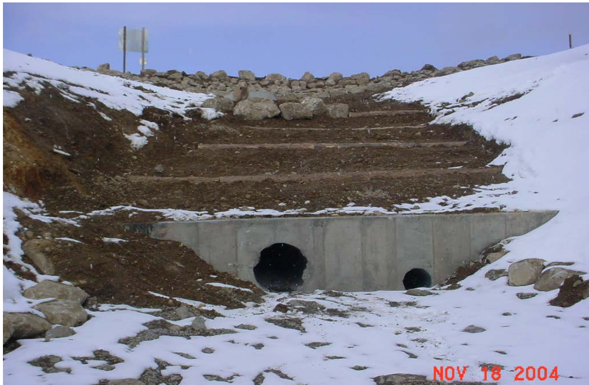
Figure 7. Erosion control structure above the pipeline headwall, November 2004 . Large pipeline is the Berthoud Pass Ditch outlet, smaller outlet is the stormwater drain for the parking lot. The stormwater drain is plugged with sediment from the parking lot and is not functioning as designed.
