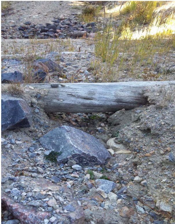
Figure 6. Rill erosion under log structure placed above pipeline headwall, September 2015.
