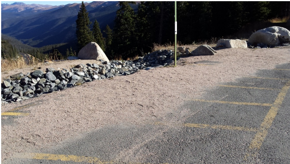
Figure 4. Sand and sediment in the parking lot just above the retaining wall, September 2015 .
