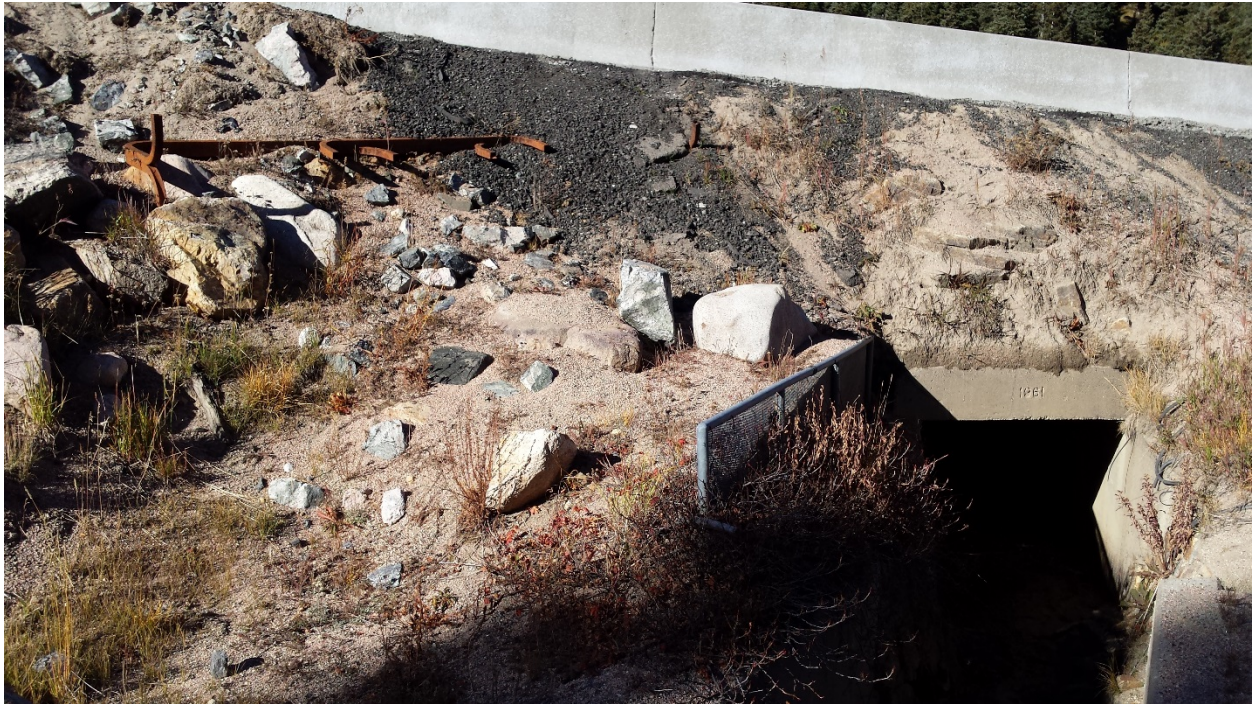
Figure 1. Deposition of sand in retaining wall along Highway 40. Rock wall above the culvert is no longer visible due to the quantity of traction sand and small fence is nearly covered, September 2015.
