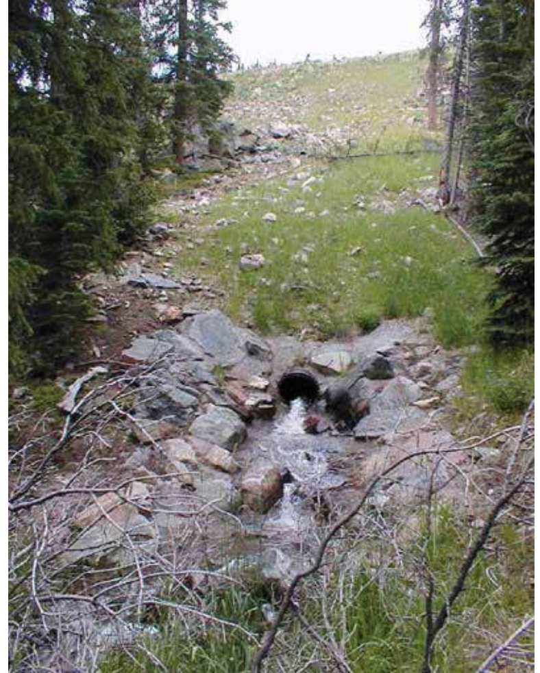
Buried Pipe Rundown
