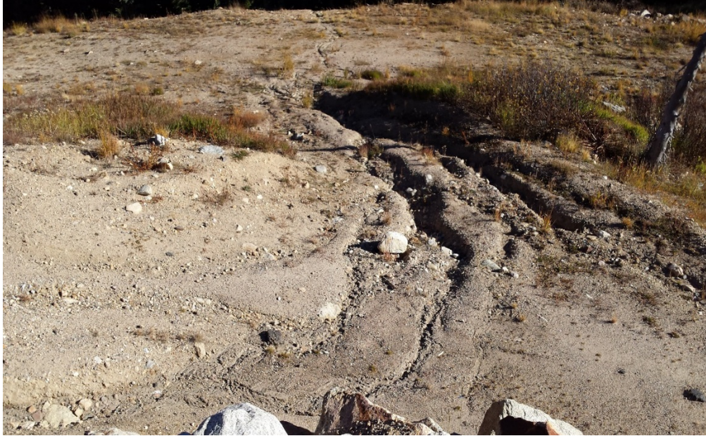
Figure 3. View of access road, September 2015 . Heavy rill erosion has made the road unstable and impassable via vehicle; retaining wall no longer visible.
