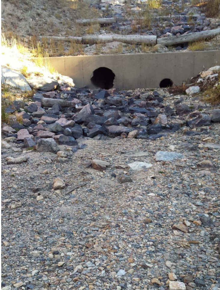
Figure 8. Sediment deposition (bottom of photo) and rill erosion above headwall, September 2015 . Figure 6 is a closeup of undercutting of log structure caused by the rill erosion.
