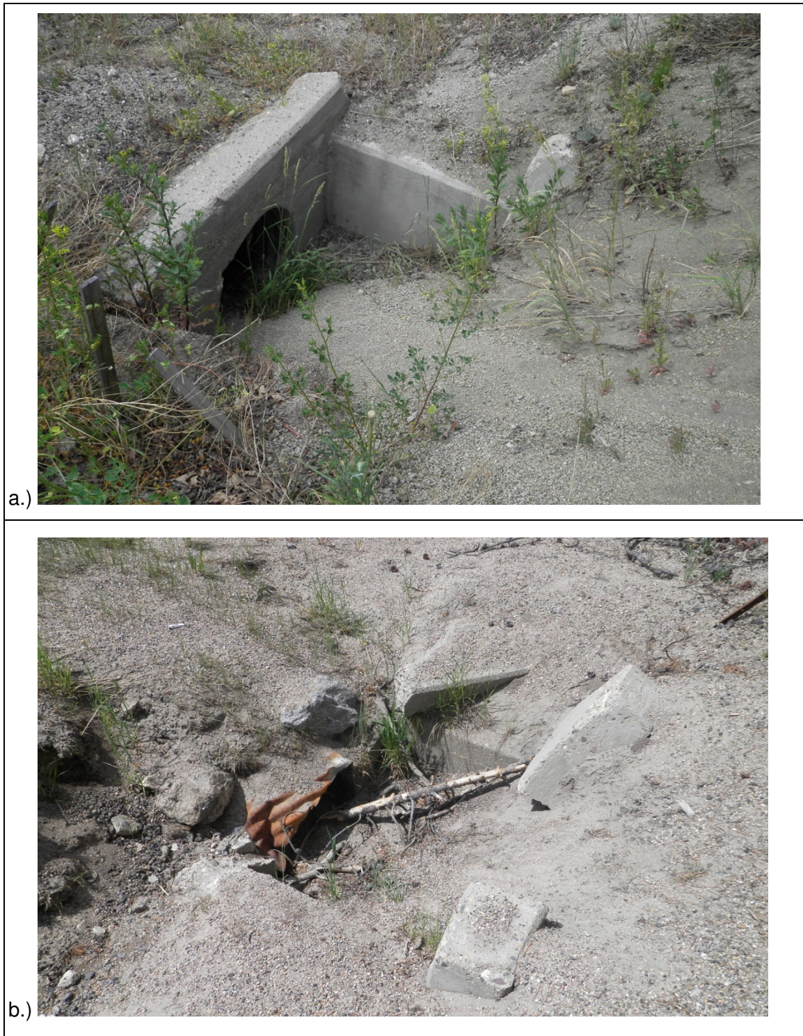
Figure 10. a., b.) Examples of partially buried and blocked culverts (MP140 and 145, respectively).
