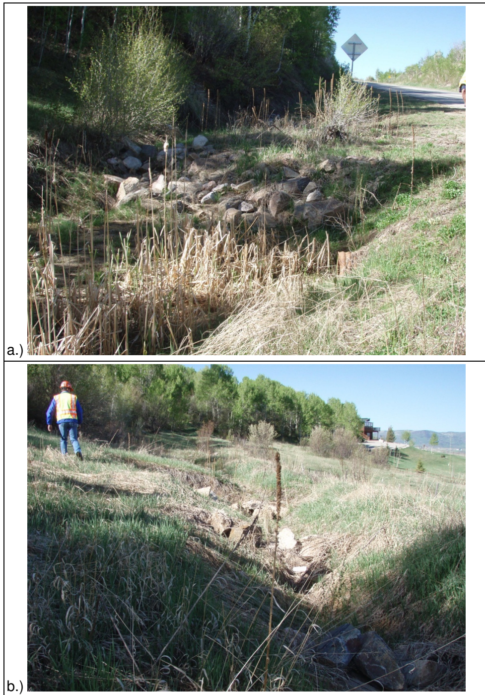
Figure 8. a.) Sediment traps placed above culvert (MP140). b.) Armored sediment traps placed below culvert outlet.
