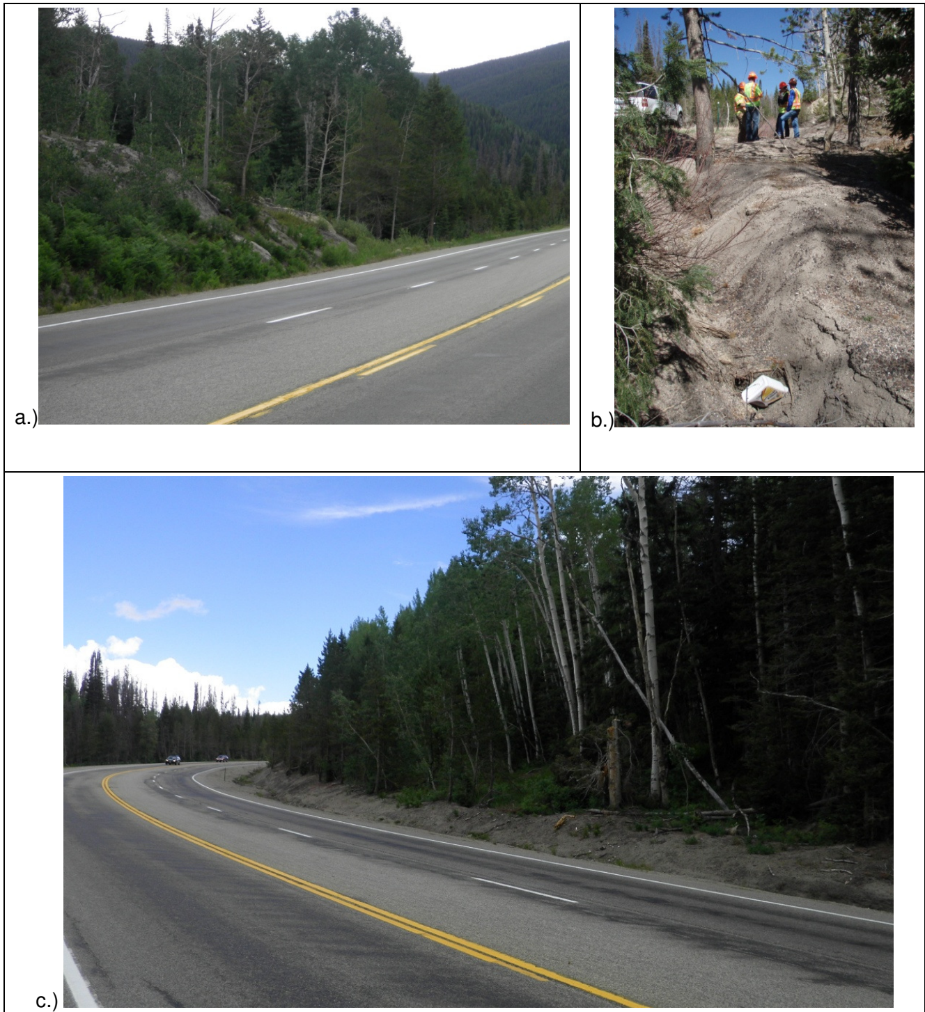
Figure 20. a.) Looking downslope, west, at section of bedrock that constrains the available space in which to implement BMPs. b.) Uphill, east, view of large deposition area located at the end of the bedrock section, depicted in (a). c.) Looking uphill, east at the channel forming along the south side of the road.
