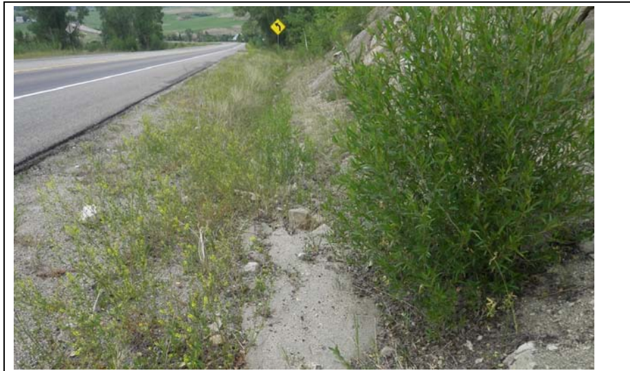
Figure 18. Looking down (north) small natural channel, just above the implemented sediment trap near milepost 140. The channel is vegetated, providing natural roughness elements that provide some control over the flows heading towards the sediment basin.
