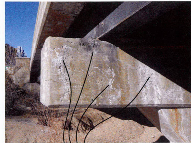
Delamination & Cracks at South Side of East Face of Pier Cap
