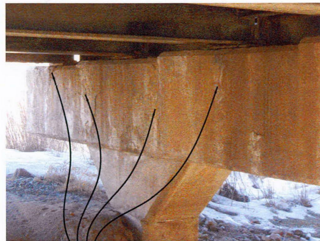
Delamination & Cracks at North Side of West Face of Pier Cap
