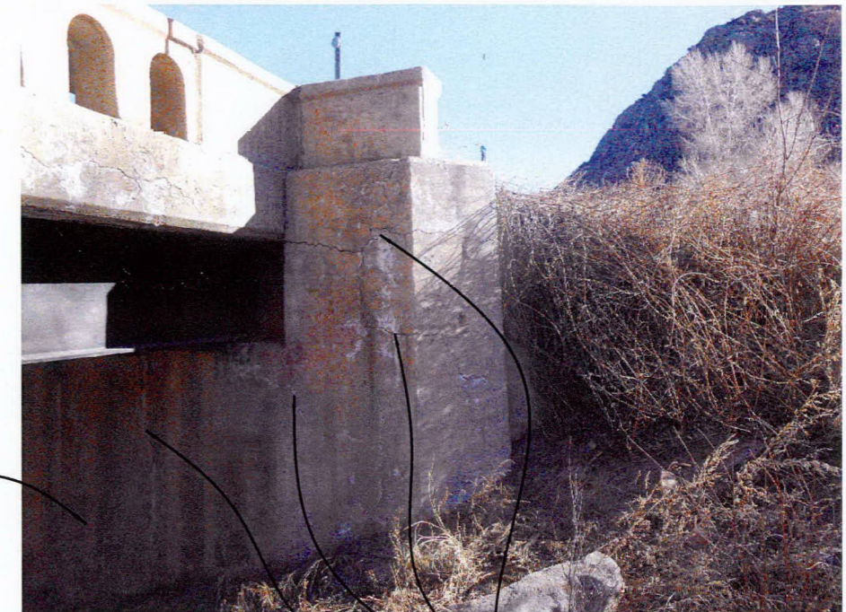
Delamination & Cracks at South Side of Abut. 3
